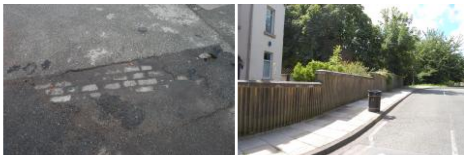
(left) granite setts beneath tarmac; (right) modern concrete slab pavements with concrete walling, presumably constructed at the time of the by-pass
