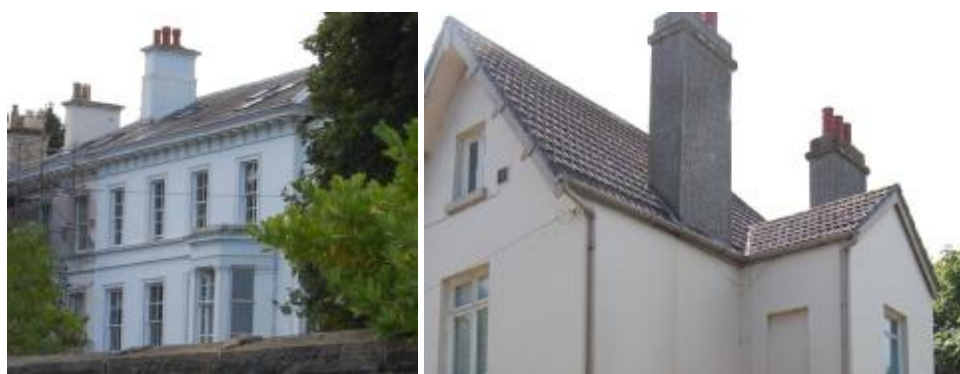
Unsympathetic alterations within the conservation area: (left) rooflights inserted into the roof slopes; (right) concrete pantiles
