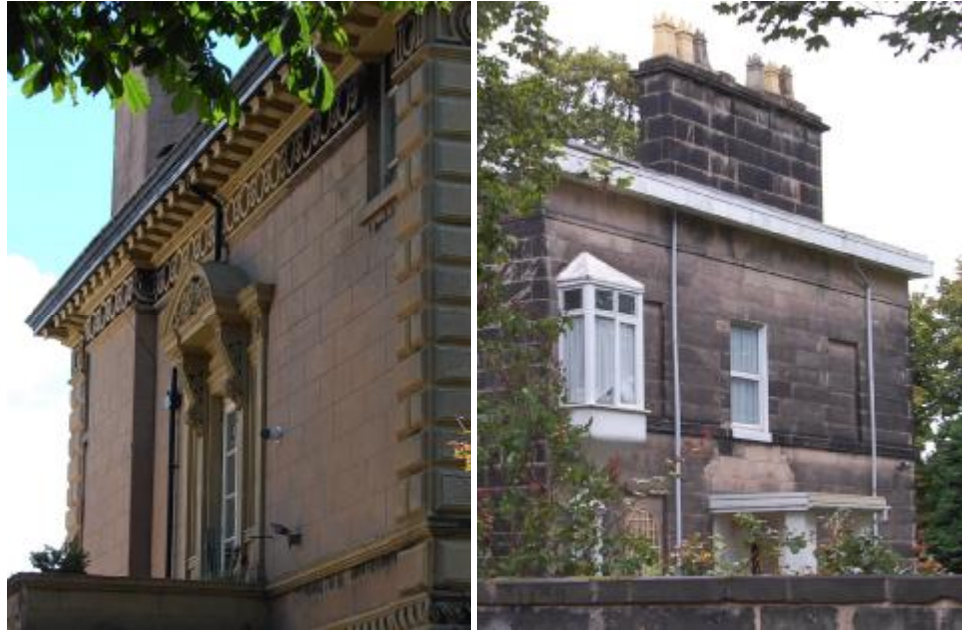
Photographs illustrating the detrimental impact of inserting new openings. The left-hand example shows a small window penetrating through the decorative cornice, the right shows an oriel window (possibly older) and a modern canopy that have unbalanced and changed the architectural quality of the façade. Both of these facades are particularly prominent.
